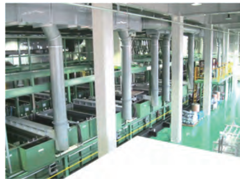
Surface treatment facility
