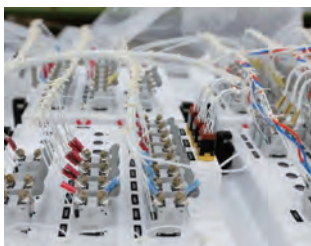
Switchboard wiring assembly
