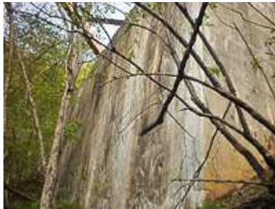
ひび割れ補修前
